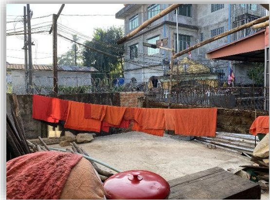
The foundation for the new kitchen, now a place to dry the longyis
