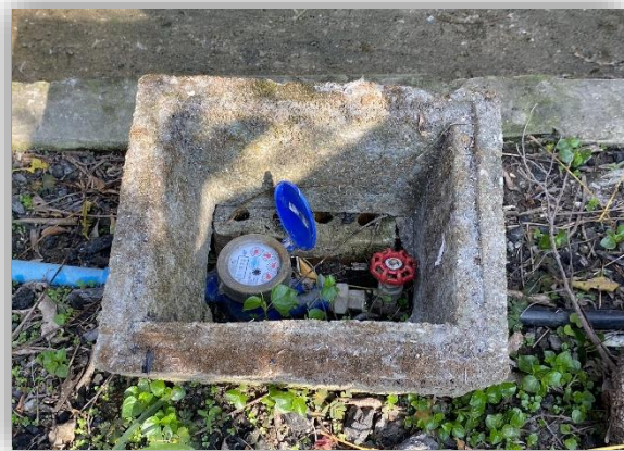
The water meter for the government water supply
